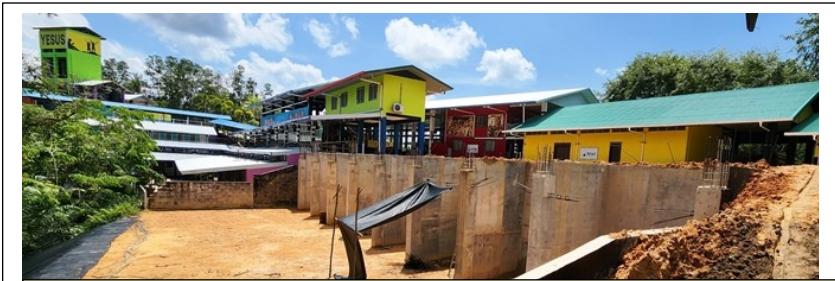
The massive foundations and first floor of our Obed building is almost completed. Getting it ready now for the second and third floors.
