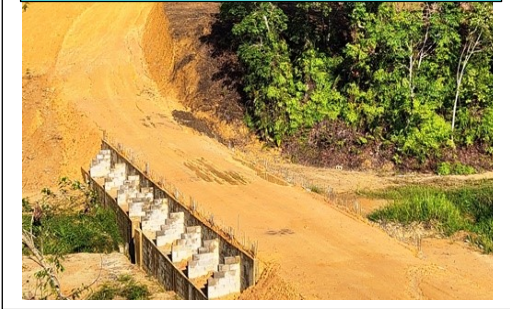
A small bridge linking up the road to our future Bible College buildings.
